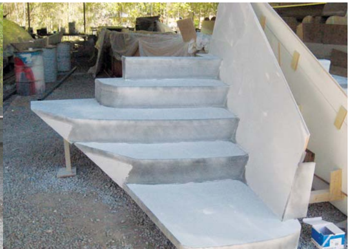
The transom steps in final stages of sanding, nearly ready for moulding.
